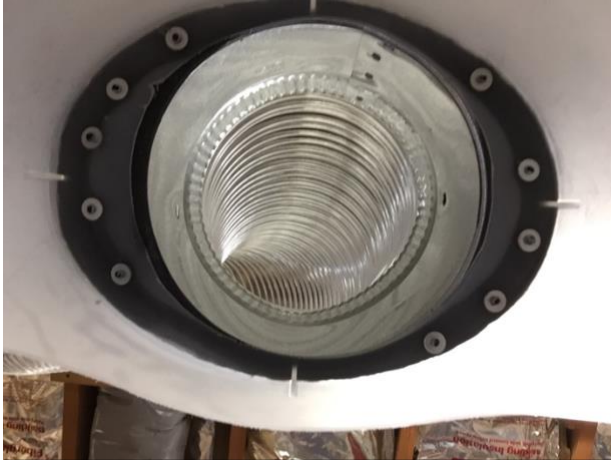
Photo 5- Inside of Dust hood showing the pop rivet washers and the black sticky foam gasket
