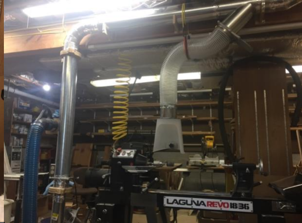
Photo 10 - Overall Picture of duct and Waste can Hood
