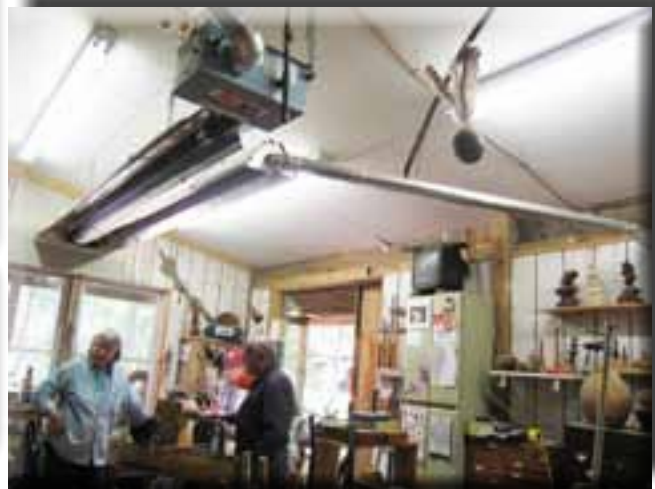
The heating system Barbara recently chose was an impressive propane radiant heater that hangs from the ceiling.
